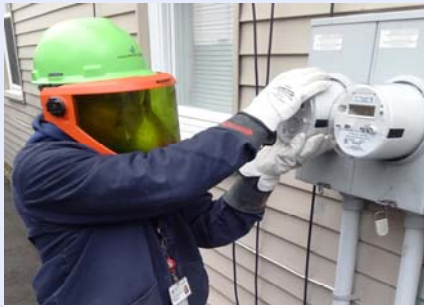
WEI Meter Installer, pictured above installing a new advanced electric meter in PMLP's service territory!
